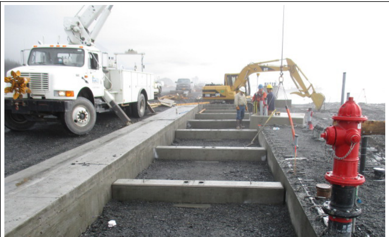
Boom truck setting a pad for electrical equipment near water services and hydrant at a ramp
